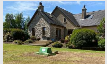
▶ Retrofit of Tricel Vitae plant
